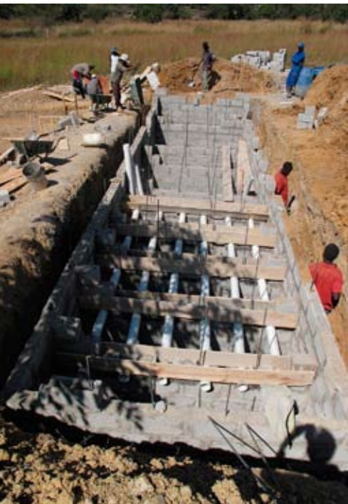
DEWATS plant with an Anaerobic baffled reactor in Zambia
